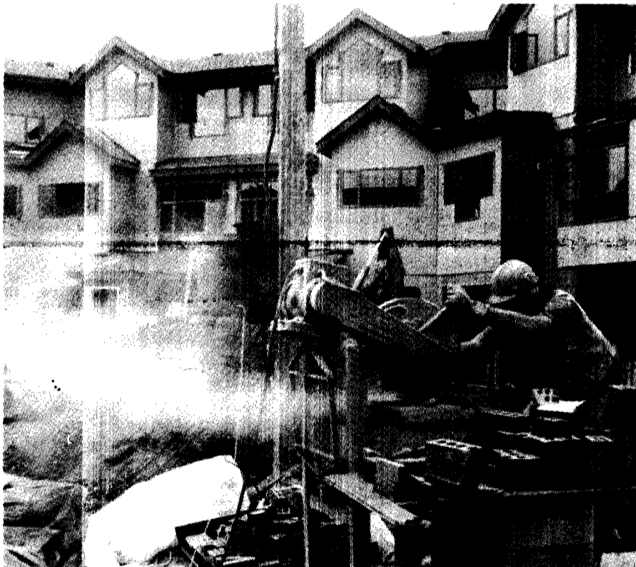
The dust is flying on the east side of the campus on Fairview Crescent just off Wesbrook Mall as workmen press on with construction of 187 townhouse units which will eventually house almost 800 UBC students. When development is completed later this year it will be leased for one year by the Expo 86 Corporation to house individuals coming to Vancouver staff international pavilions at the 1986 world exposition. Total cost of the new housing development will be about $14.3 million.
