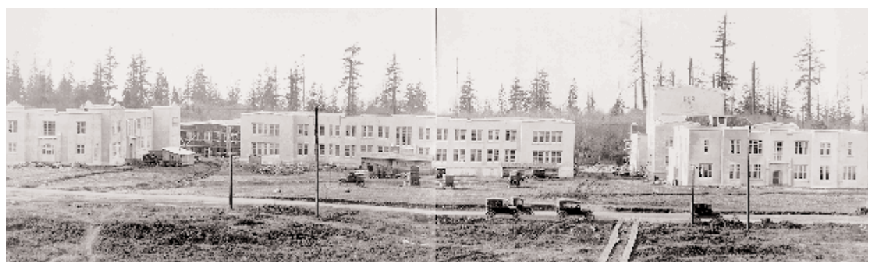
Semi-permanent buildings (left to right, Agriculture, Arts, Auditorium, Administration) under construction. Dogged by financial constraints in 1925, nine buildings, all of wood-frame and stucco construction were classed as "semi-permanent" and designed to last 25 to 40 years "if necessary." (As of 1996, most were still in use.) □
