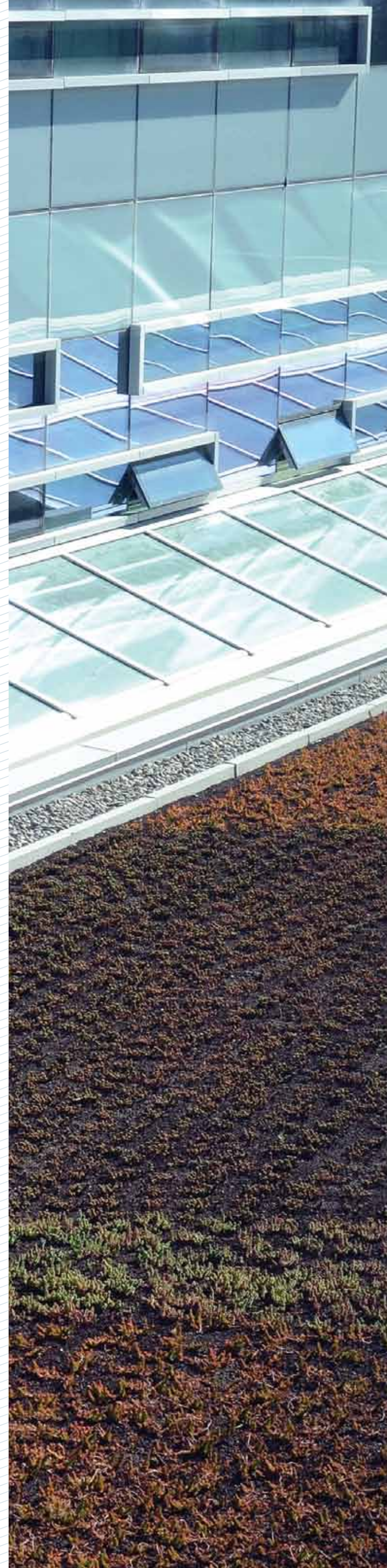
Okanagan Campus green roofs provide natural temperature control.
